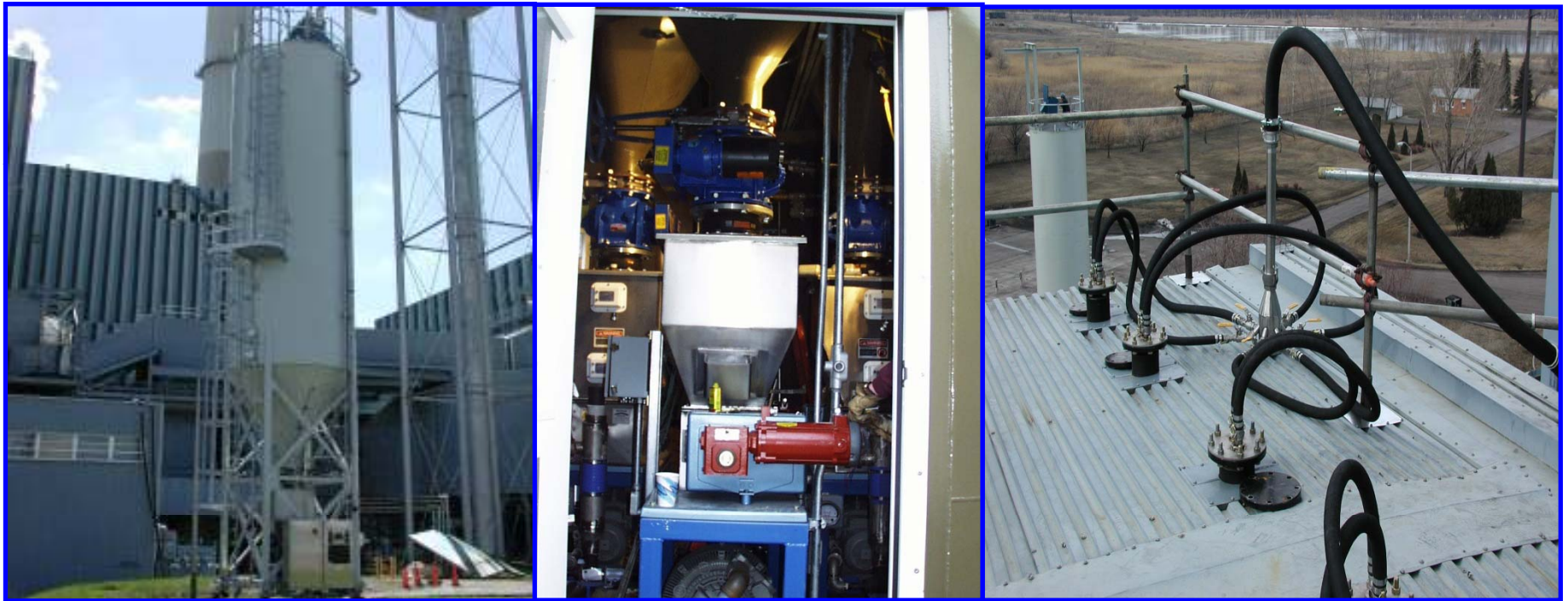
• PAC Storage Silo
